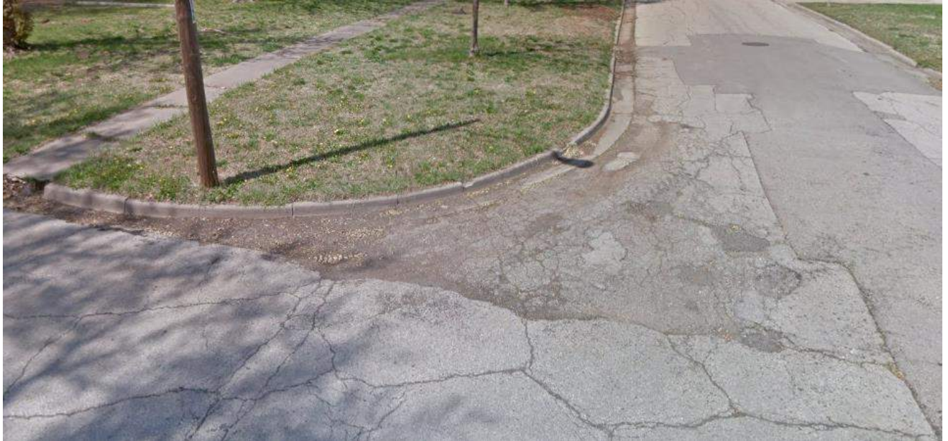
Figure 3-5: Results of Ponding
