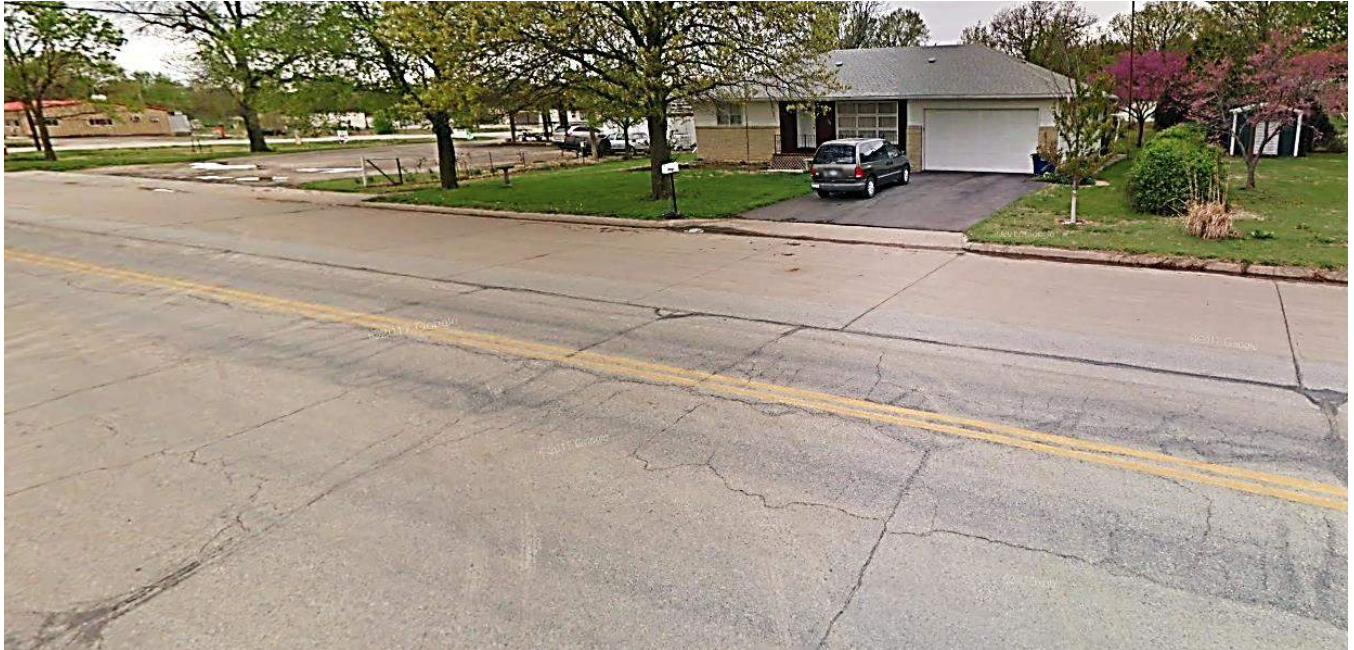
Figure 2-12: Example of “Fair” Condition – North Jefferson Street
