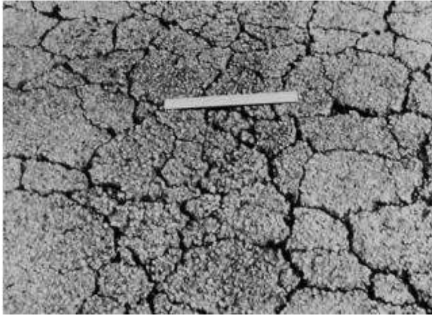
Figure 2-3: Example of Alligator Cracking (ASTM)
