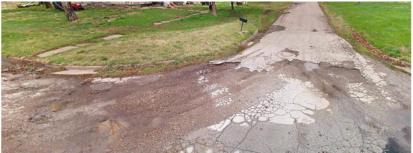
Figure 2-14: Example of “Very Poor” Condition – East 6 th Street.
