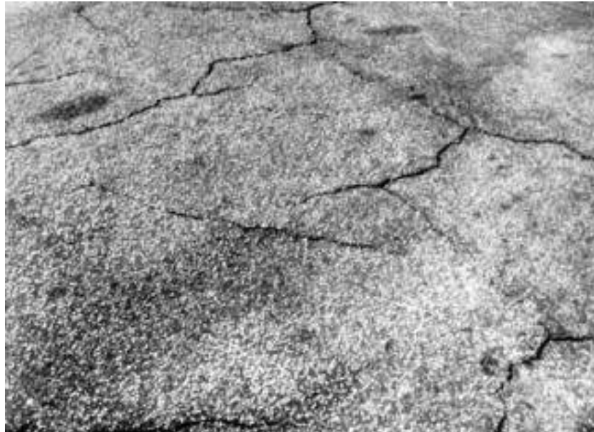
Figure 2-4: Example of Block Cracking (ASTM)
