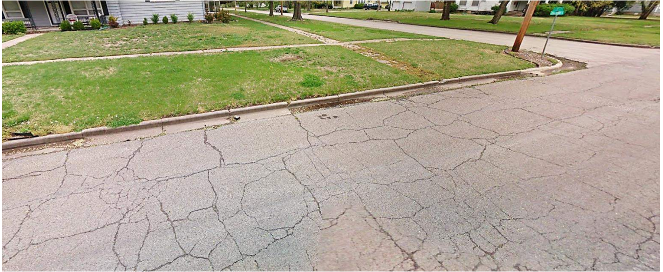
Figure 2-13: Example of “Poor” Condition – North Mulberry Street
